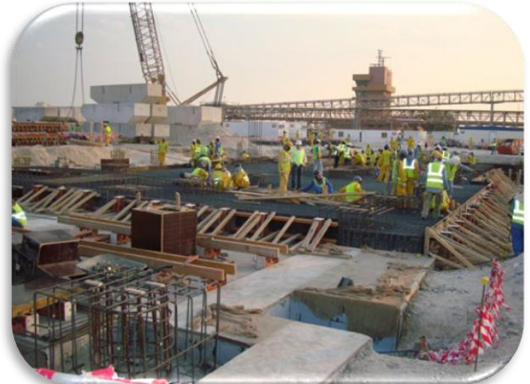
Berth 7 Substation Building STFA/QP – DOHA/QATAR
