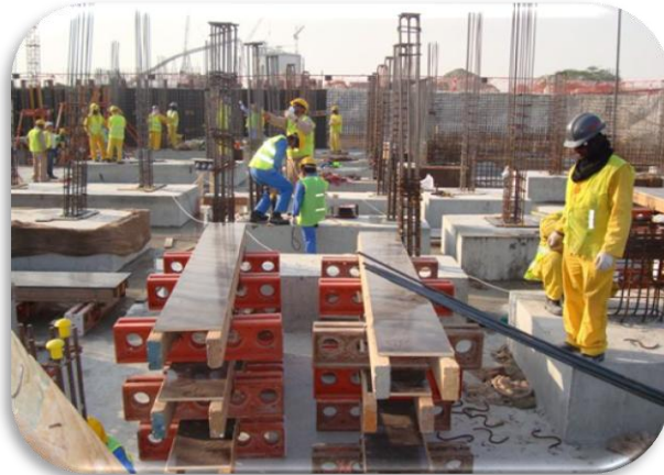
Berth 7 Substation Building STFA/QP – DOHA/QATAR
