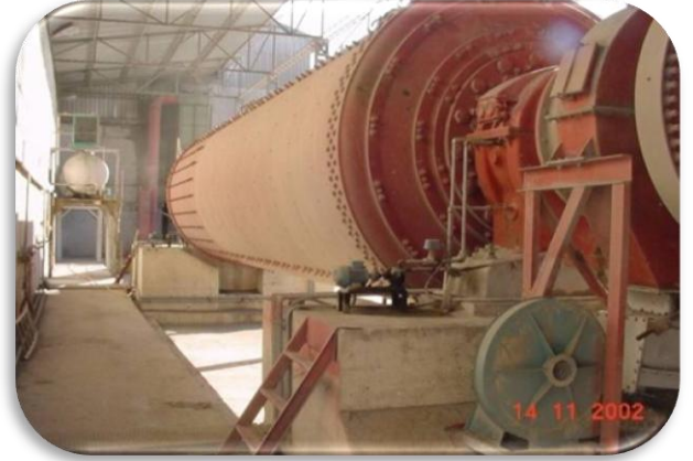
Cement Grinding Plant – GEBZE/TURKEY
