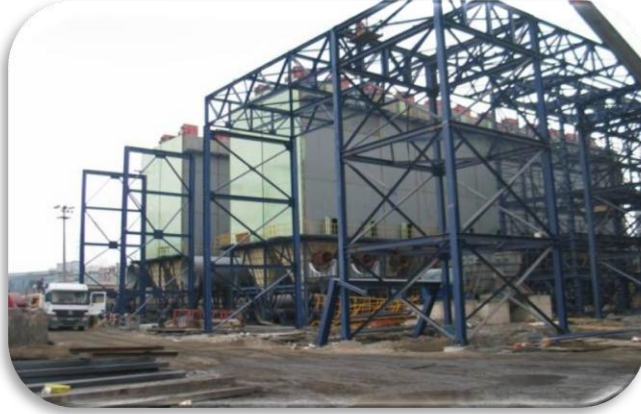
Co Generation Plant – KOCAELI/TURKEY
