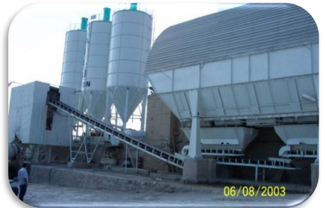
Ready Mix Concrete Plant – TUZLA/TURKEY
