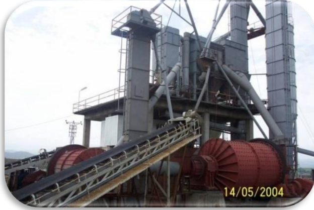
Calcite Grinding Plant for Power Plant – ÇAN/TURKEY
