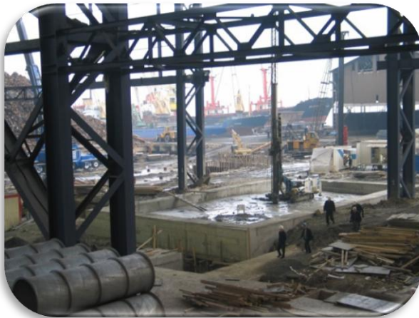
Water intake scale pits
